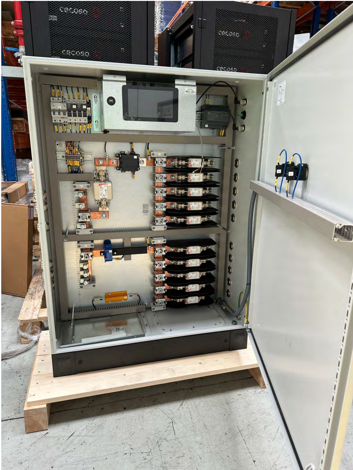
Figure 16. Inside of PCC of power battery
