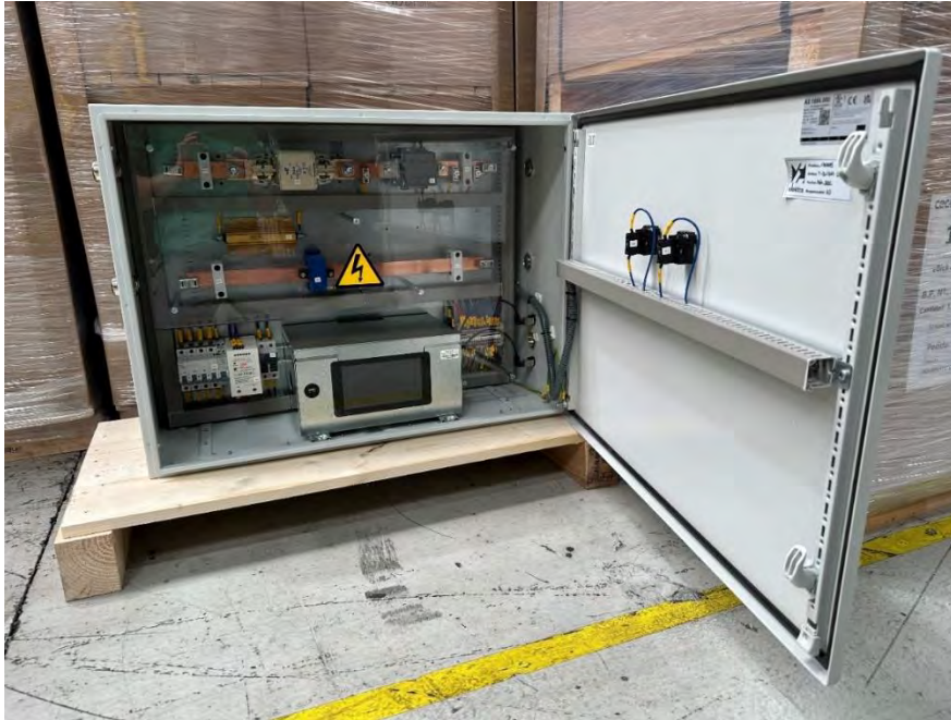
Figure 3. Inside of PCC for high-energy battery
