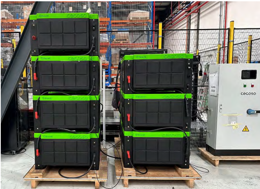
Figure 4. Validation of the high-energy battery pack
