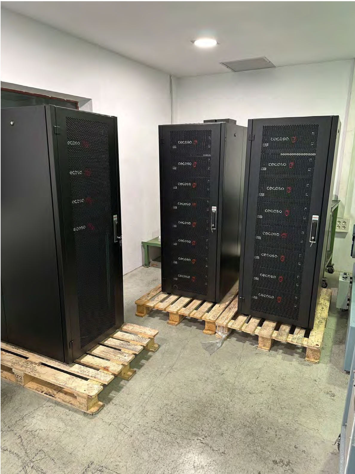
Figure 14. High-power battery cabinets
