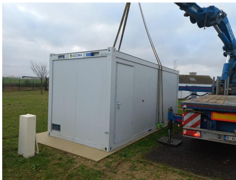
Figure 1. Installation of the iSTORMY container at the Concept Grid laboratory
